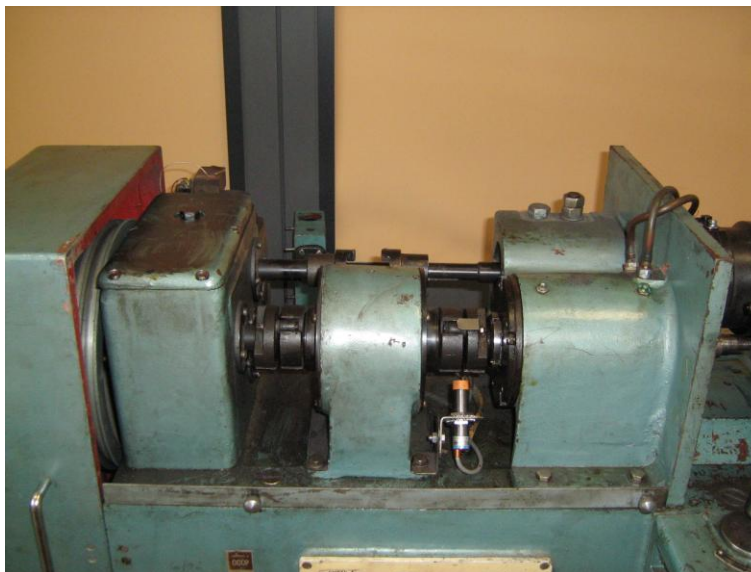
Fig. 4.3.3.3. A view of the carriage drive shaft after removing the cover. Visible pipes for cooling water supplied from the water supply system
