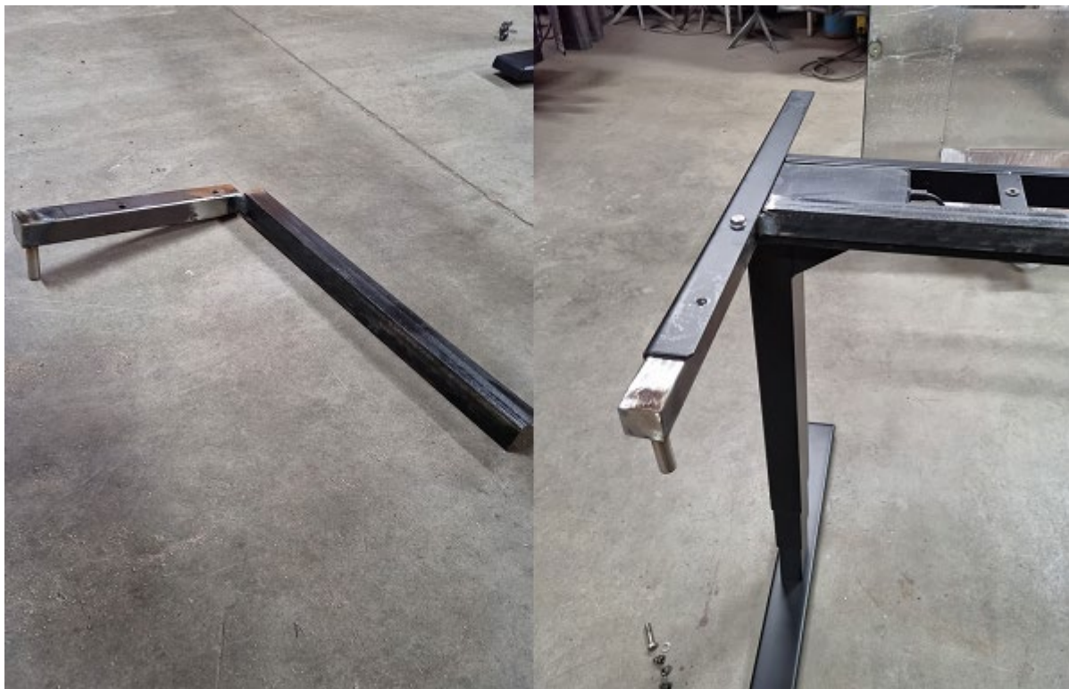
Fig. 39. Mounting the arm for the welding table control panel on the ERB-1 frame
