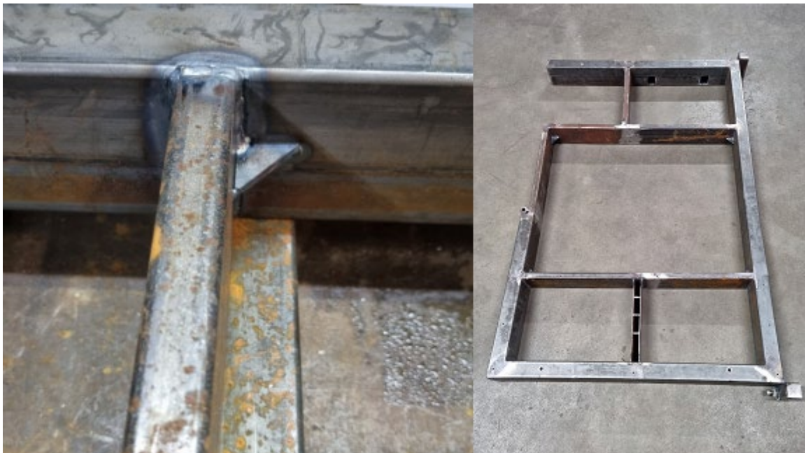
Fig. 36. Making welded joints of 80x20x2 profiles of the truss frame separating the ventilation space of the lower exhaust from the space for tool storage
