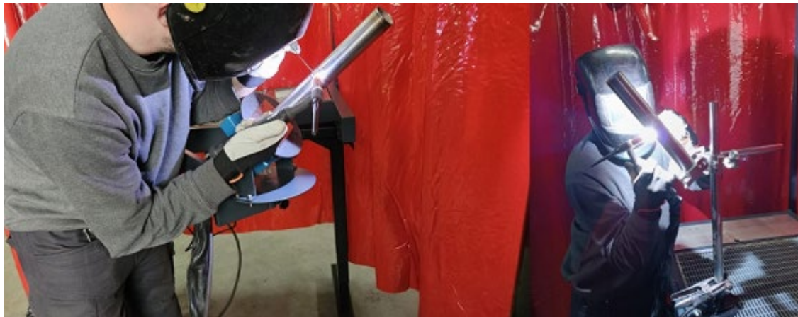
Fig. 55. Operational test of the designed and constructed welding table. TIG welding of a pipe in the HL-045 position using a turntable
